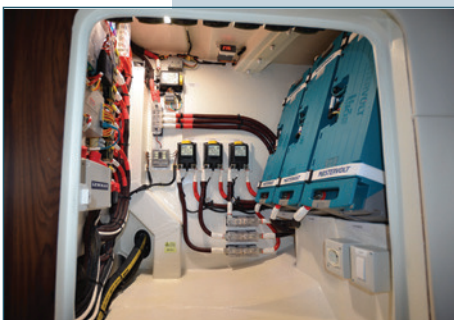
An electrical technical compartment on each side: a specific customer request.
